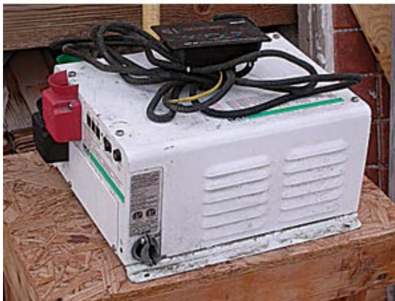
These six-volt 186 amp/hour batteries and this old 4000-watt Trace inverter came from scrapped RVs.
