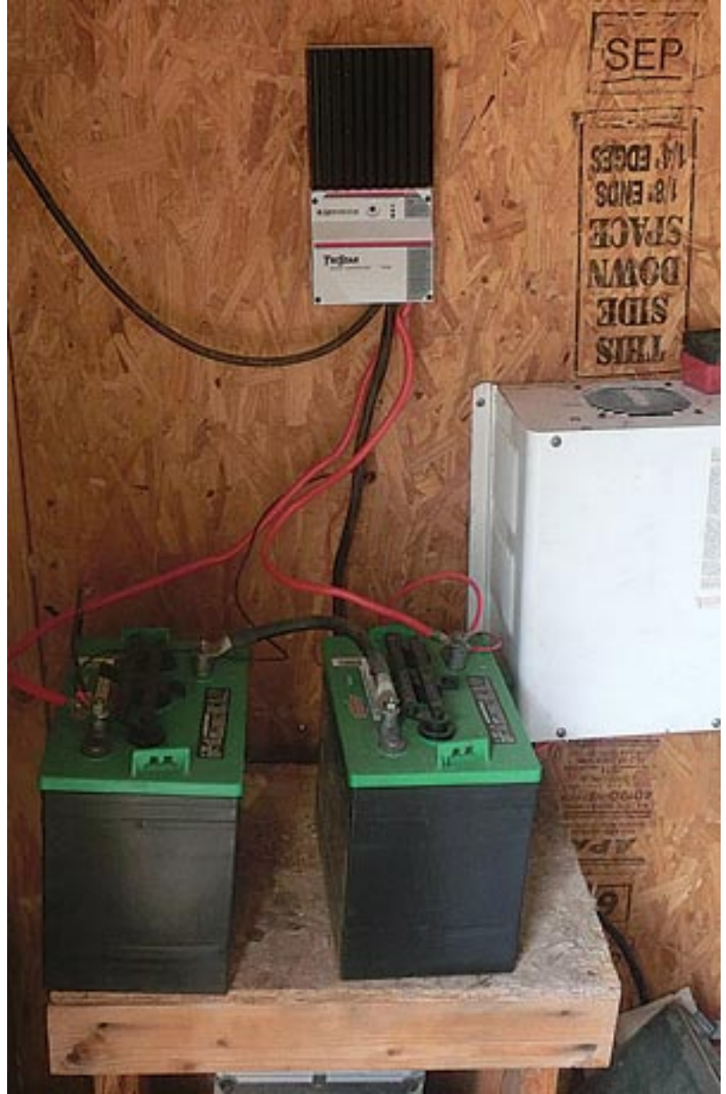
After about 18 months I replaced the scrounged batteries with these two new Interstate 230 amp/hour batteries.
