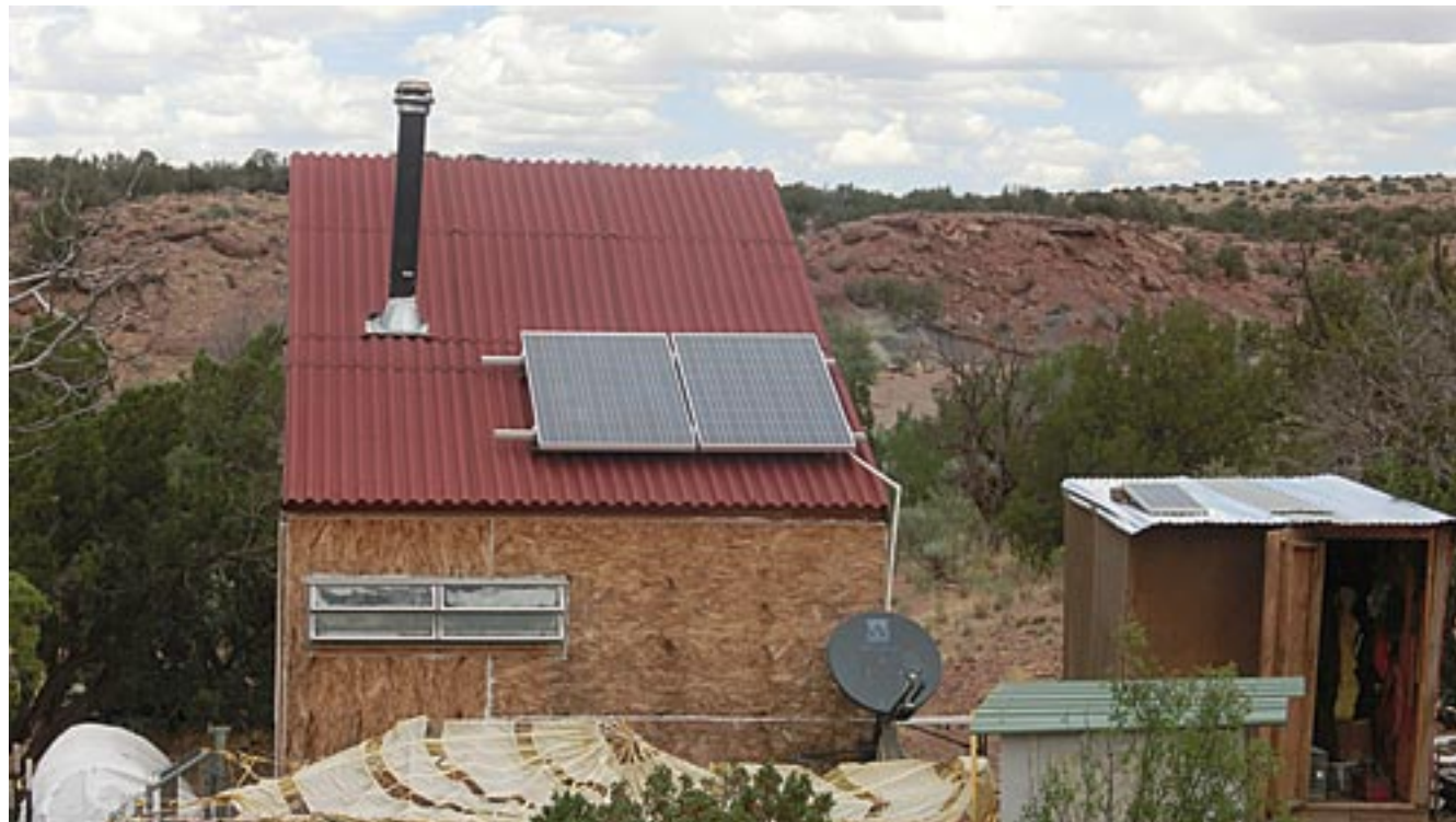
The solar panels are installed on my south-facing roof.
